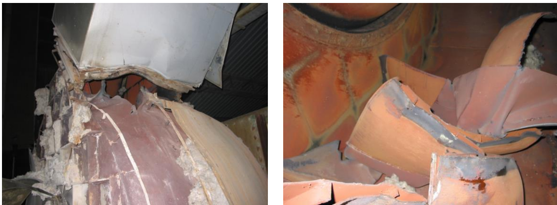
Fig. 3. Failure in a fan.
